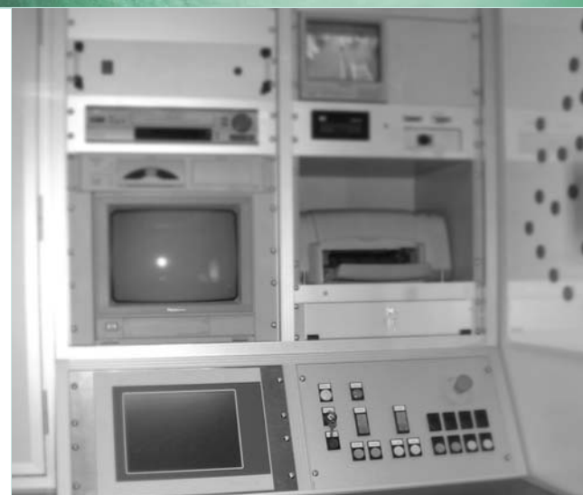
The control panel enables the user to control the curing process down to the last centimetre.
